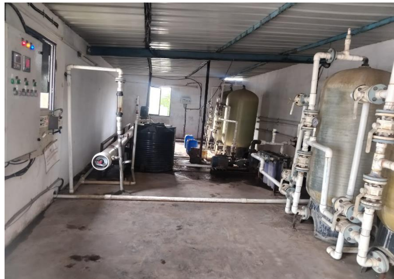
R.O. Facility at the plant premises
